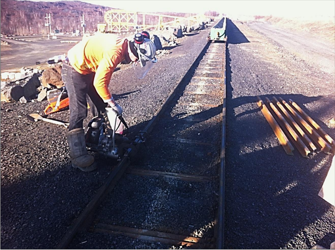
Figure 3-9: A healthy section of rail being removed to introduce a faulted section (shown on the right).
