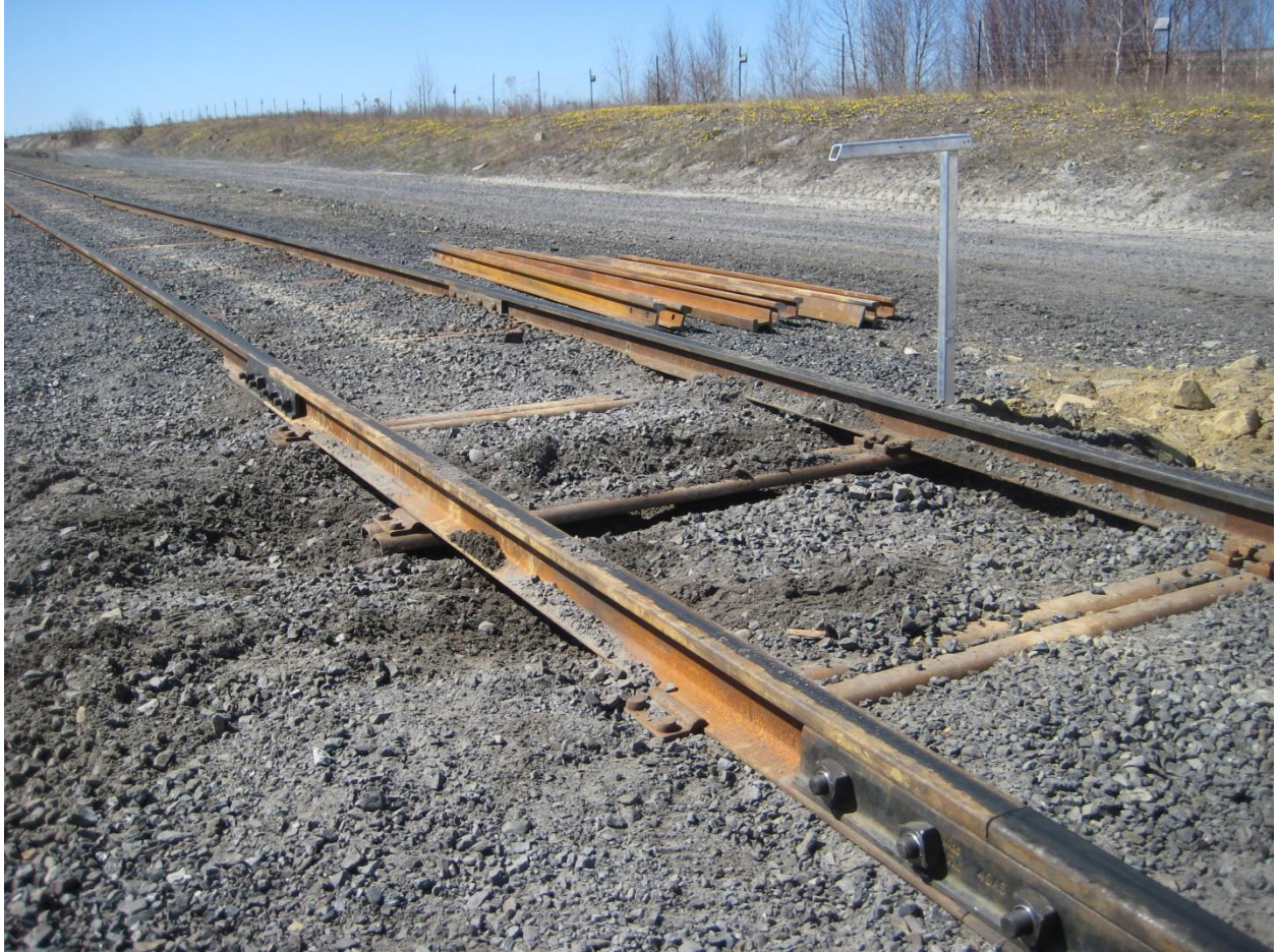
Figure 3-14: The experimental setup of the slight washout with 30 mm crack in the base.
