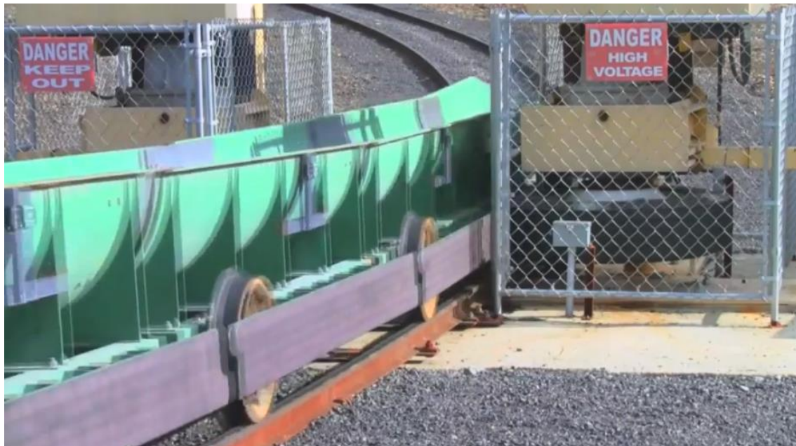
Figure 1-1: The Rail-Veyor® train passing through a drive station (taken from [3]).
